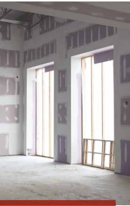
Energy-efficient insulation is layered behind drywall in the new Fostoria 7-12 School building expected to open in January 2020
