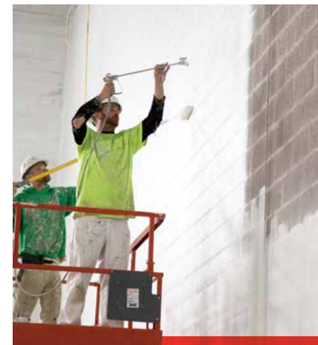
Members of the construction crew apply finishing touches to a new wall at the new building
