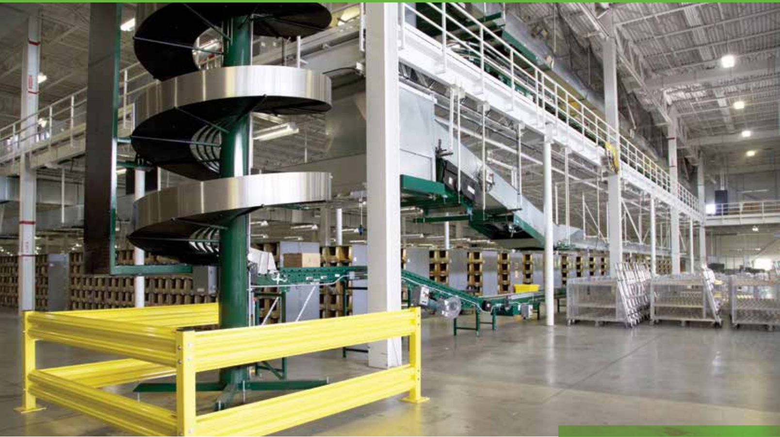
Abercrombie's conveyor belt system in Distribution Center 2 is optimized for energy efficiency
